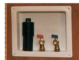
Residential washer/dryer hook-up in laundry closet.
