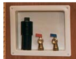
Residential washer/dryer hook-up in laundry closet.
